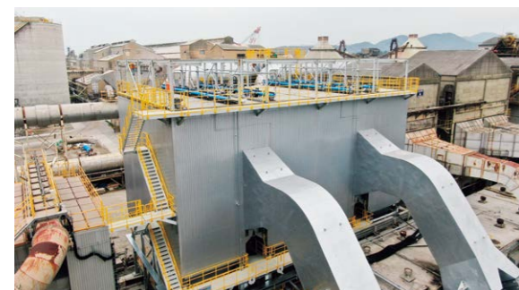
Ako Plant: Switching from electrostatic precipitators to bag filters
