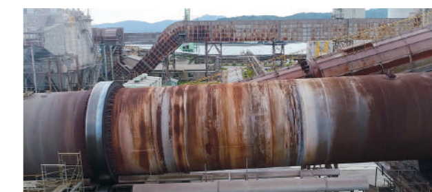
Rotary kiln (Aiko Plant)
