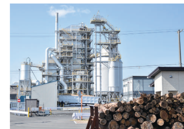
Hachinohe Biomass Power Generation Co., Ltd. (Hachinohe City, Aomori Prefecture, Japan)
